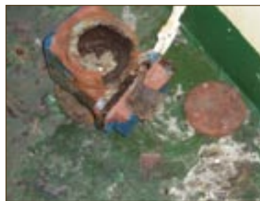
Defective vent head
