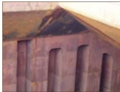
Crack in topside plating
