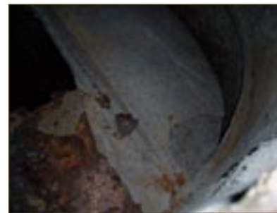
Defective engine room fire damper
