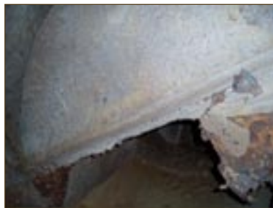
Defective engine room fire damper
