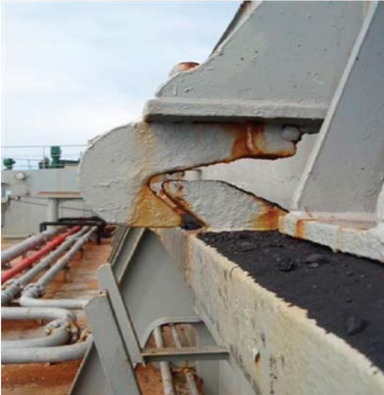
Hatch securing arrangement – excess clearance means no positive securing forces
