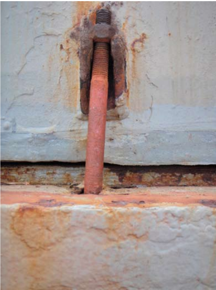
Hatch cover as found, in fully closed position and secured. Note lack of sealing
