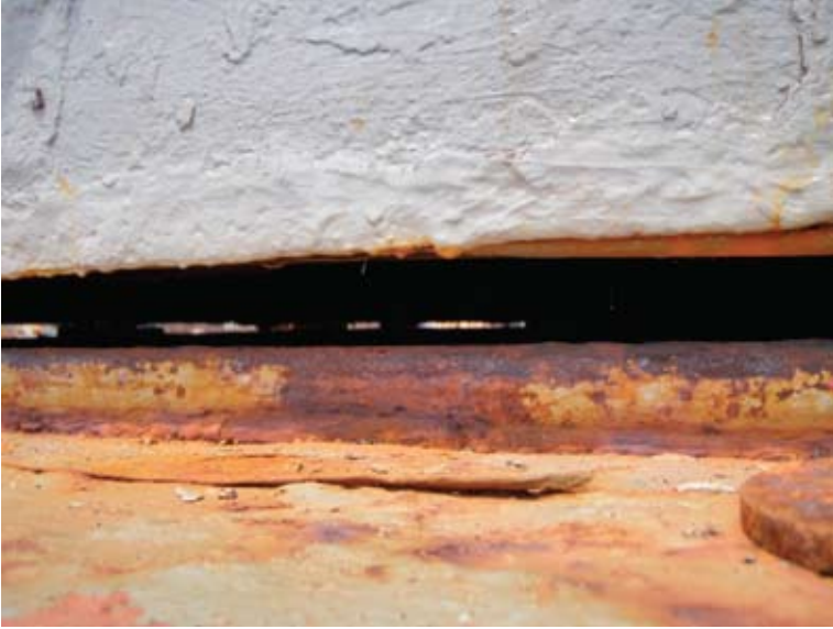
Hatch cover as found, in fully closed position
