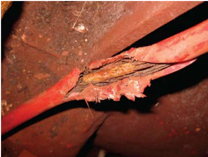
Lifeboat release cable conditions
