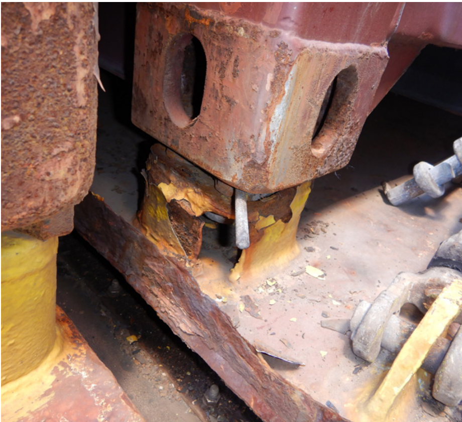
Corroded and cracked raised ISO socket.
