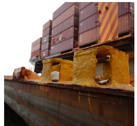
Corroded raised ISO sockets.
