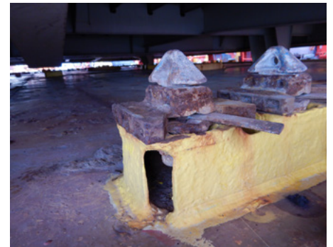
Corroded raised ISO sockets.
