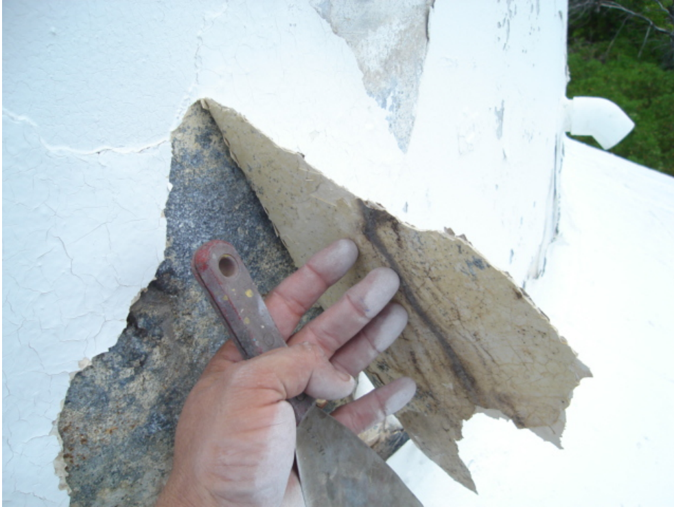
Condition of tower paint system – test showing adhesion
