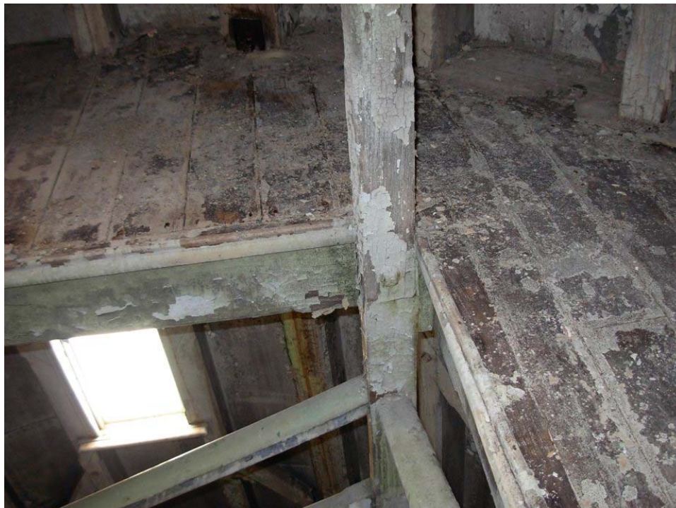
Condition of internal paint system
