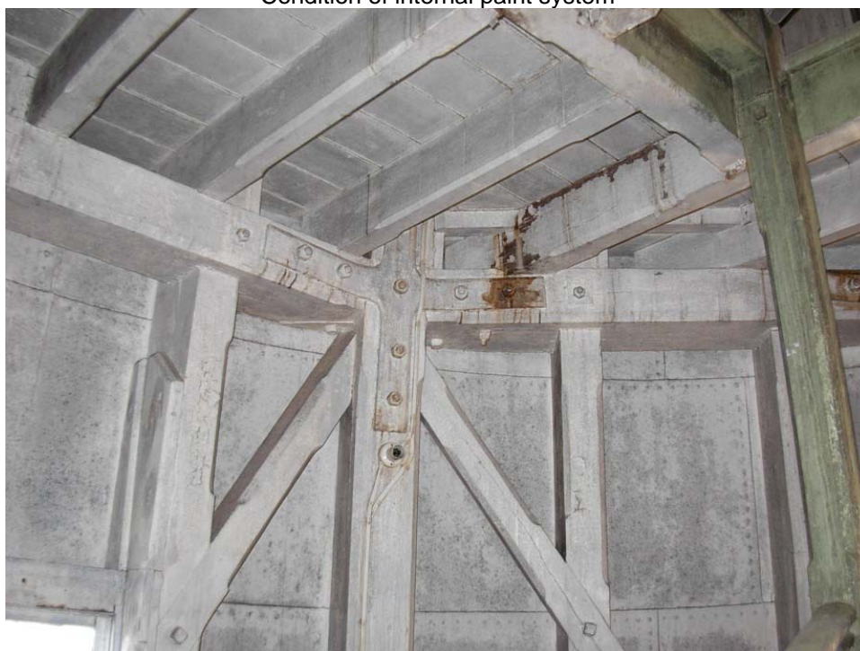
Condition of internal paint system
