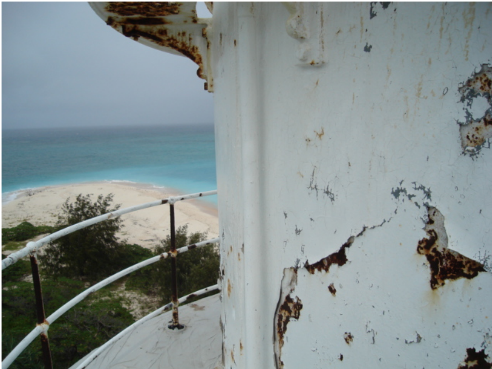
External corrosion and paint system
