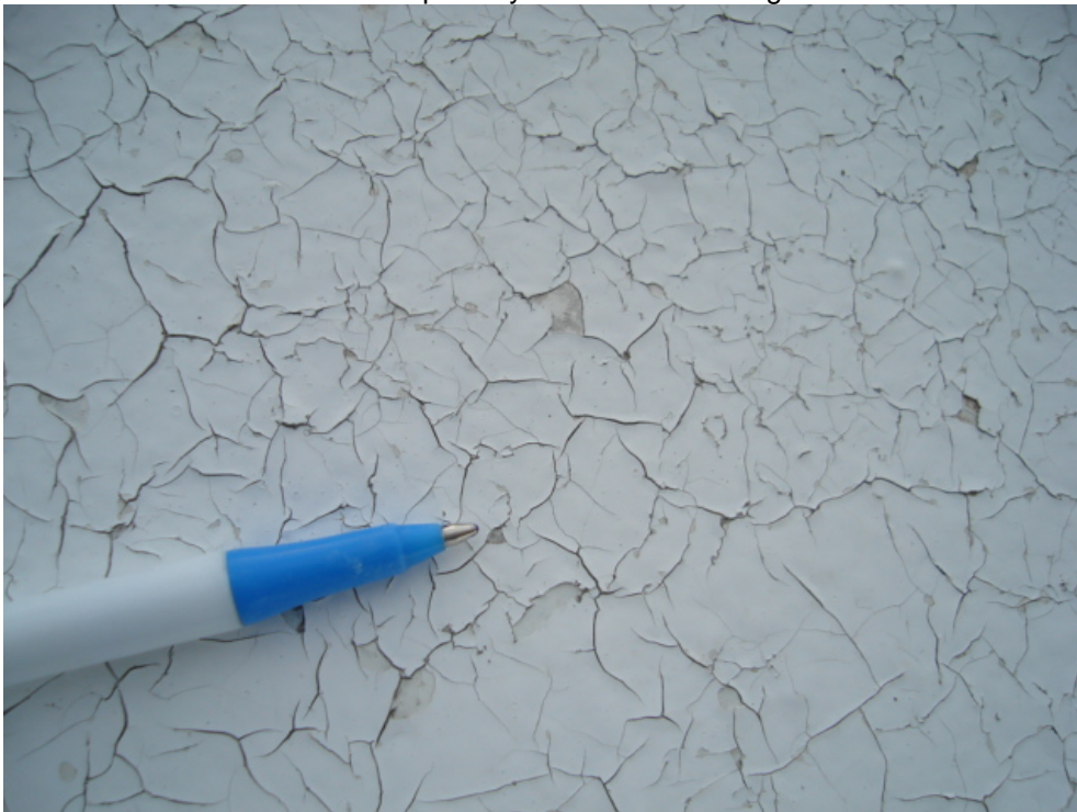
Condition of tower paint system
