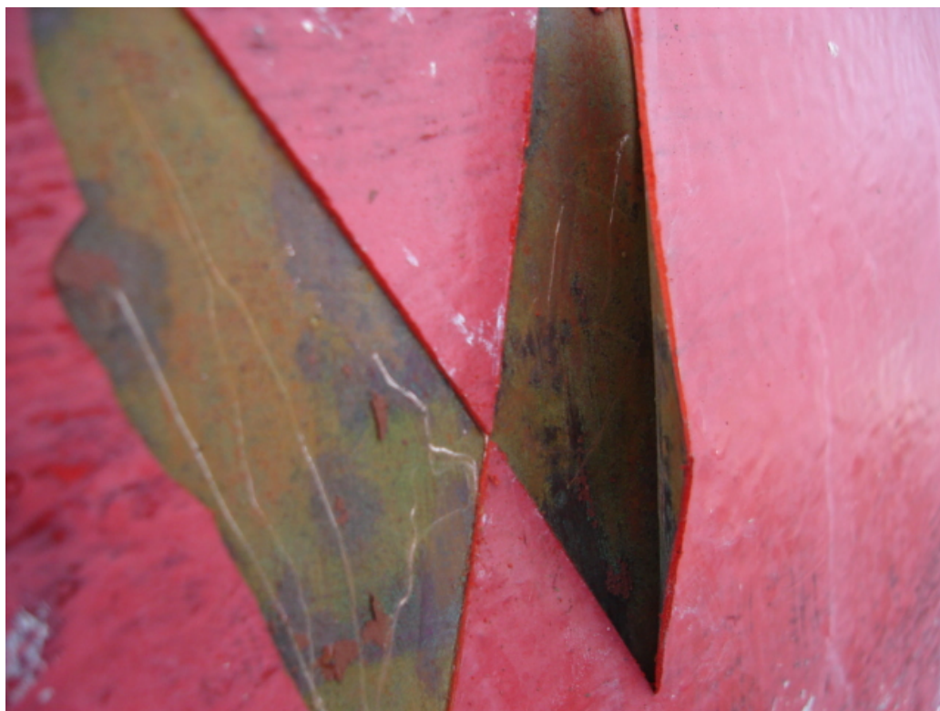
Condition of dome paint system – test showing adhesion
