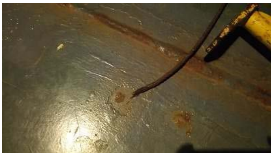
Parted wire from unapproved secondary means of support
