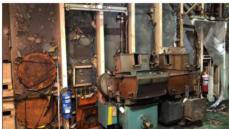
Case study 2 – Heat damage to engine room forward bulkhead
