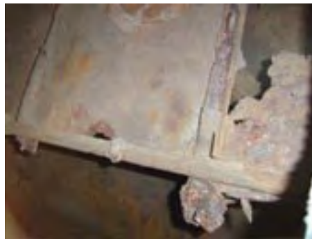
Defective engine room fire dampers
