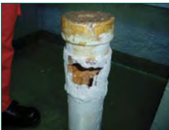
Corroded sounding pipe
