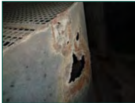
Heavy corrosion of ventilators
