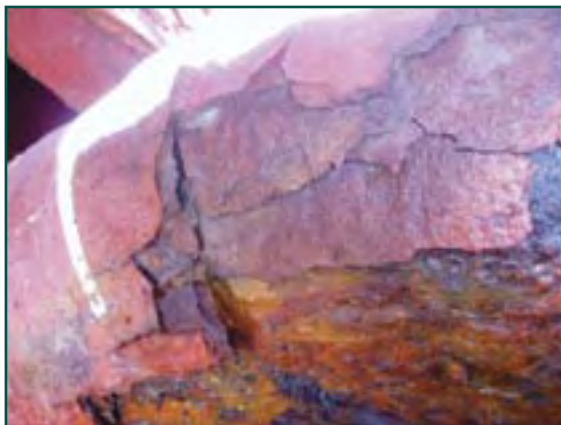
Heavily corroded fire main
