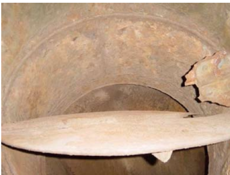
Detached engine room fire damper
