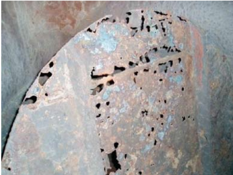
Defective engine room fire damper
