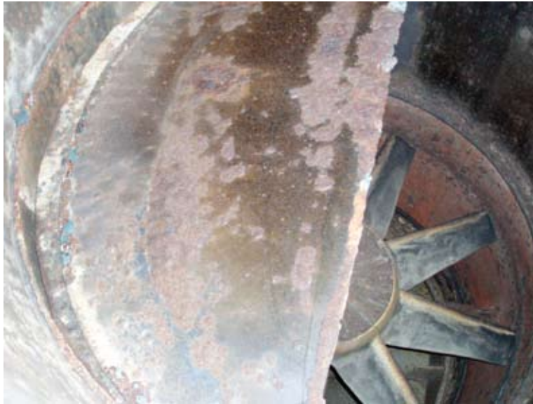
Defective engineroom fire damper
