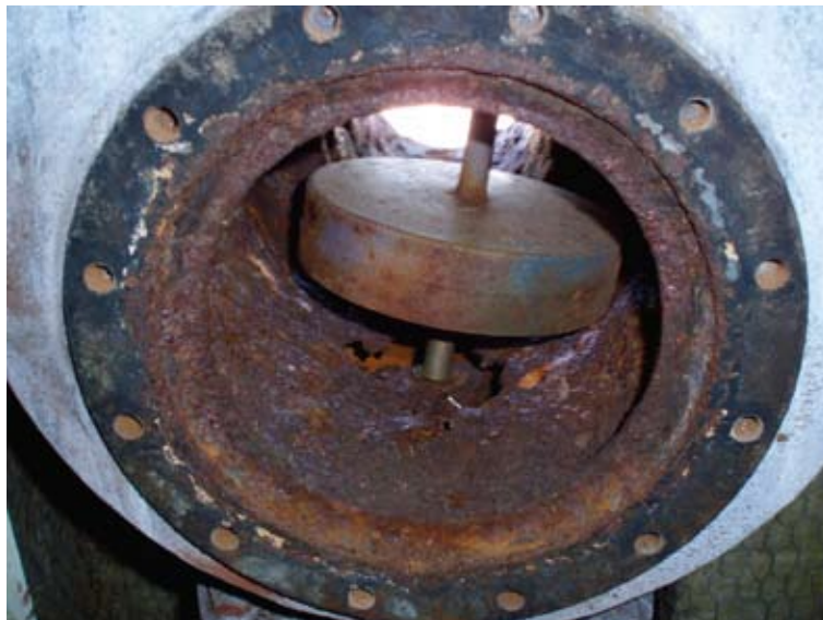
Defective tank air pipe
