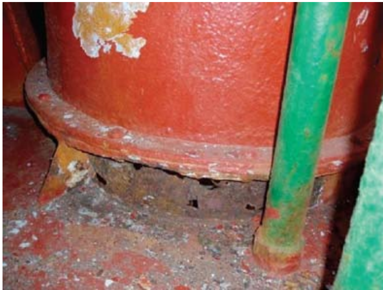
Defective damper ducting
