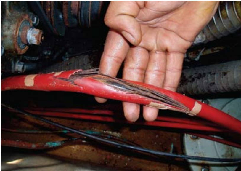
Defective operating cable for lifeboat release arrangement
