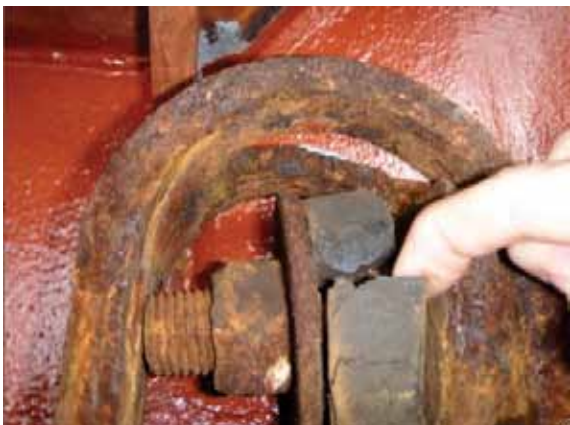
Damaged hatch cleat
