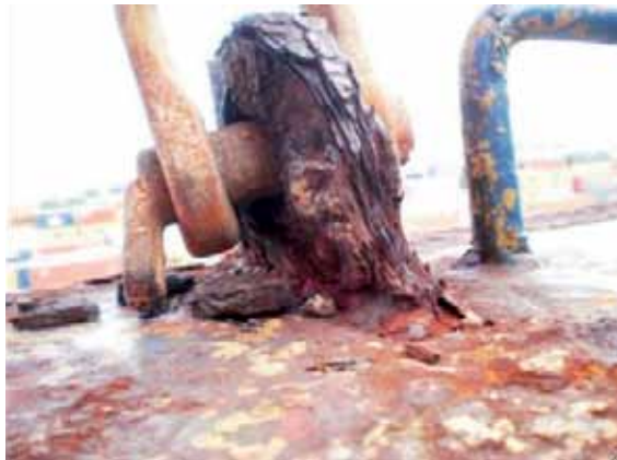
Corroded lashing plate
