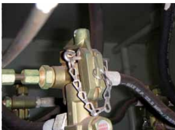
Fixed CO 2 system transportation safety pins still in place
