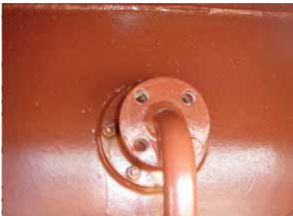
CO 2 pipeline to cargo hold flange not connected
