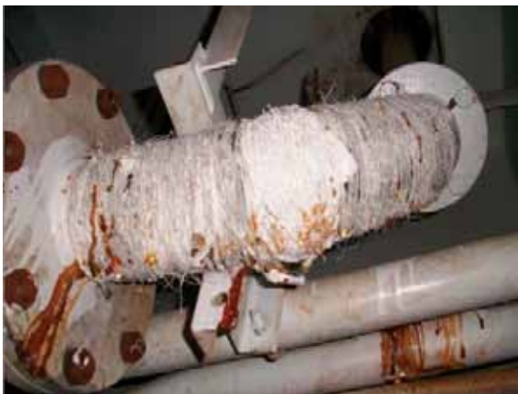
Holed sea water pipe
