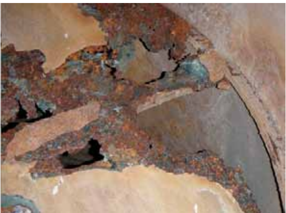
Fire damper wasted and holed
