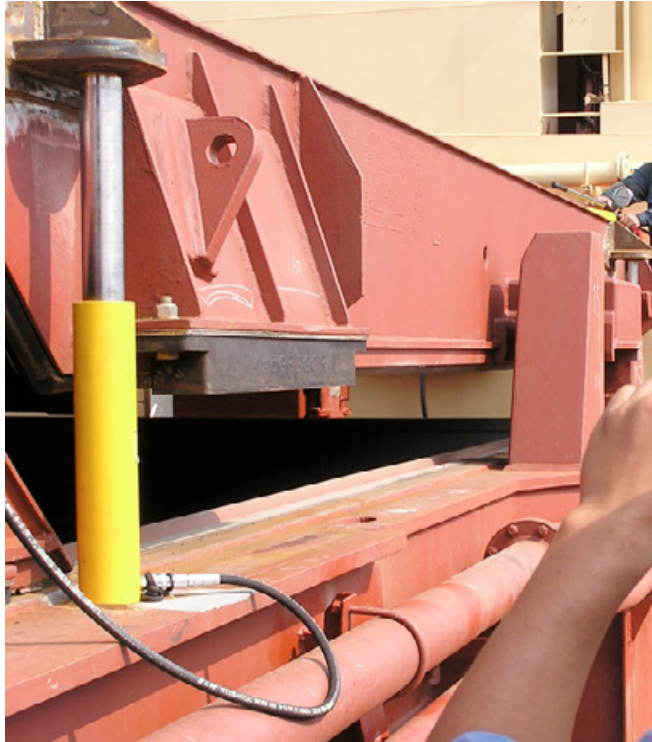
Hatch cover jacking arrangement
