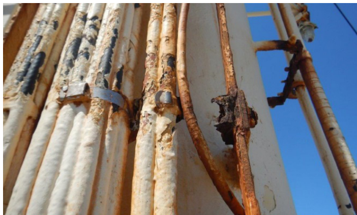
Figure 9: Wasted cable trays on main navigation mast (source: AMSA)
