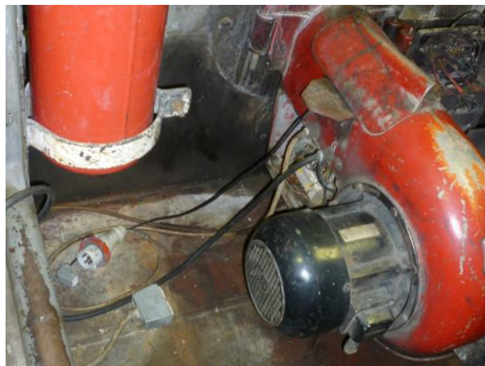
Figure 4: Restricted working space where the engine rating had to work (source: Transport Malta)
