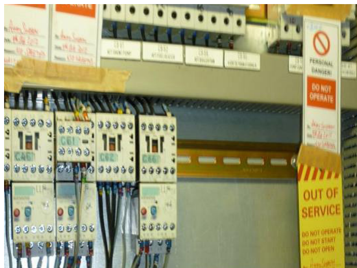
Figure 3: Safety tags on the circuit breakers (source: Transport Malta)
