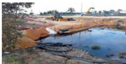
Western side of South Road - road works material bunding oily waste
